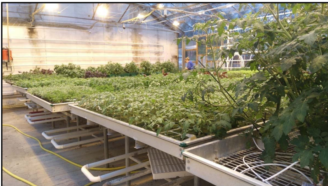
Figure 5.8: Heating pipes under the plant benches, on the side of walls in an Icelandic greenhouse.
