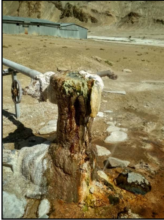
Figure 1.11: The condition of one of the wells at Puga (June 2019). This well was used to heat the poultry farm and the mushroom farm which can be seen in the background. The geothermal fluid was directly circulated in pipes inside the sheds for heating.
