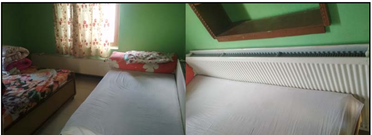
Figure 1.28: Radiators installed in the guest room in Chumathang as part of demonstration project.
